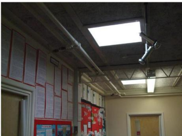
Picture 9- Block 11 Uninsulated old heating pipework (D1)
