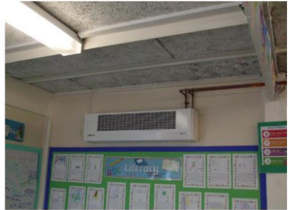
Picture 8- new fan convector (typical classroom) in Block 11 with old heating uninsulated pipework to be replaced with new (D1).
