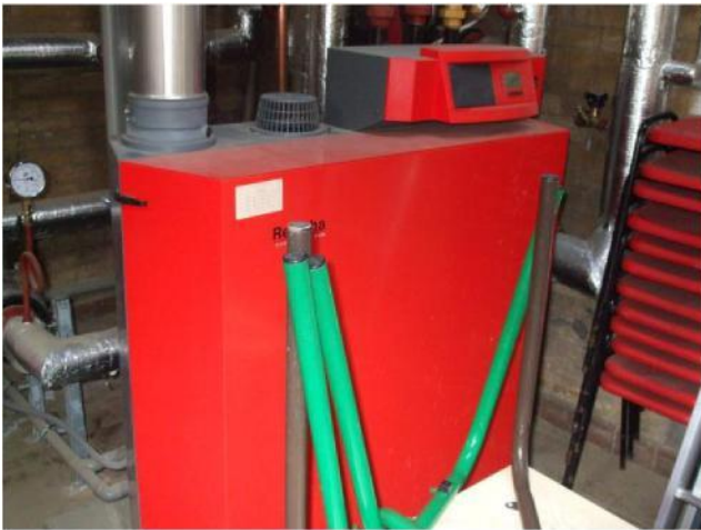
Picture 11- Boiler No 2 in Block 11 plantroom In good condition (A4) 11-GF-155
