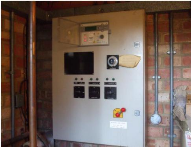
Picture 5- Existing control panel to be (12-GF-171) (D1) Replace with new.
