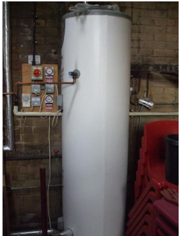
Picture 14- Block 11 cylinder to be retained in plantroom 11-GF-155 (B2).
