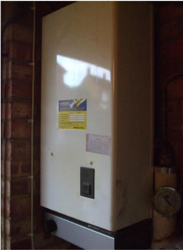
Picture 1- Existing Boiler 12-GF-171 Plantroom (D1)
