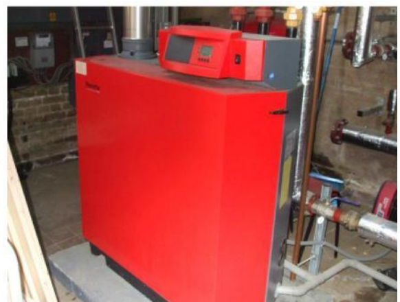
Picture 10- Boiler No 1 in Block 11 plantroom in good condition 11-GF-155 (A4)
