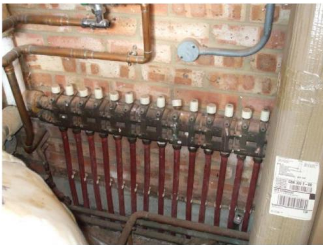
Picture 3- Underfloor heating manifold in 12-GF-164 Plantroom (B4)
