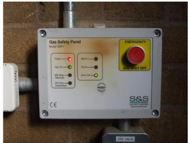
Picture 12- Existing gas safety control panel 11 plantroom 11-GF-155 to be replaced (B2)
