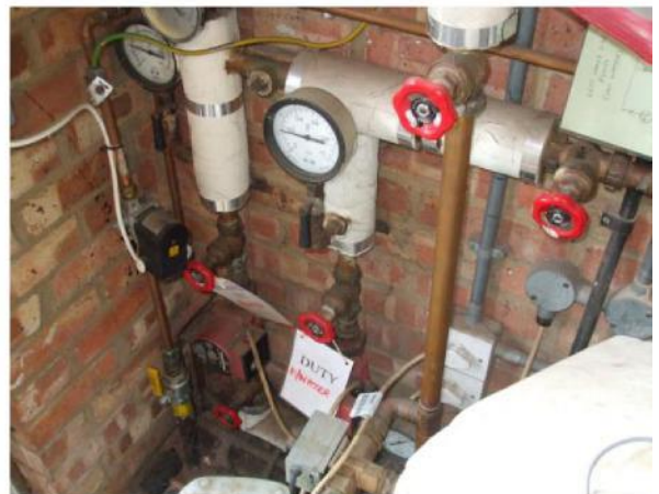
Picture 4- Grundfos single main heating primary pump (D1) in 12-GF171 Plantroom
