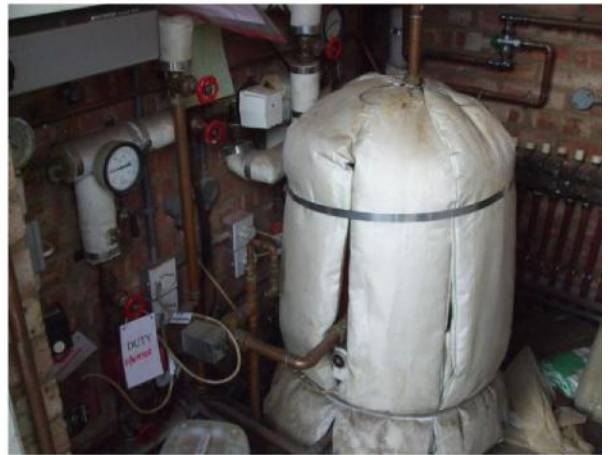
Picture 2- Existing cylinder 12-GF171 Plantroom D1
