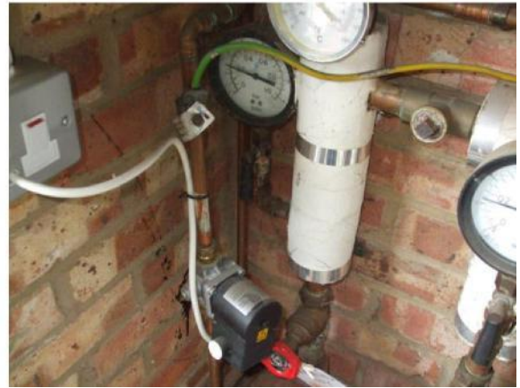
Picture 6- Gas solenoid valve to be replaced with new in 12-GF-171 Plantroom (D1).
