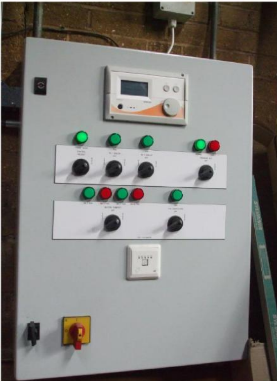
Picture 13- Existing mechanical control panel in Block 11 plantroom 11-GF-155 in good condition (B4)
