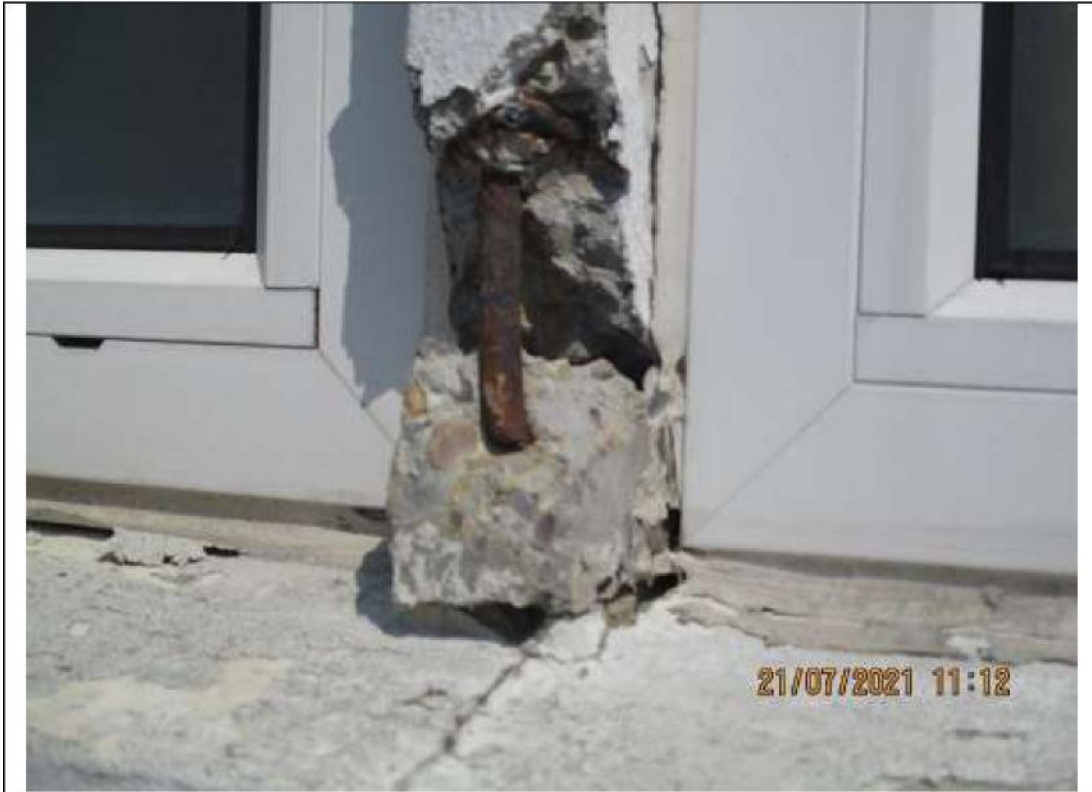
51) Example of defective concrete surround to windows.
