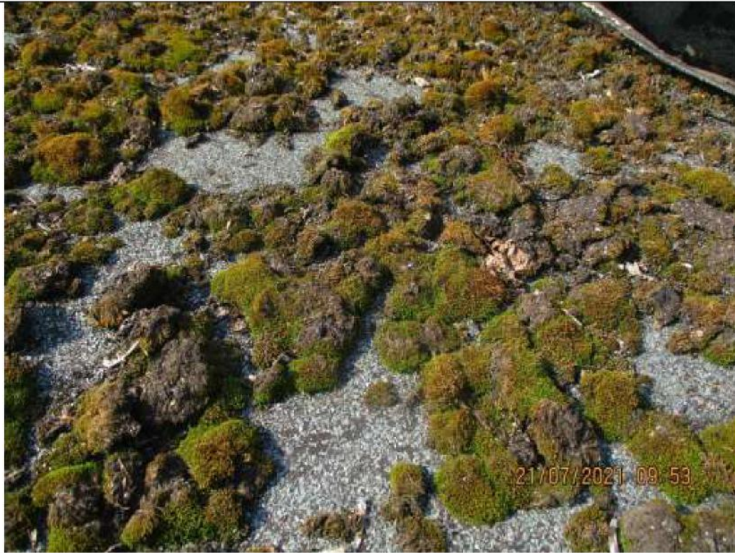
19) Build up of moss growth to flat roof.
