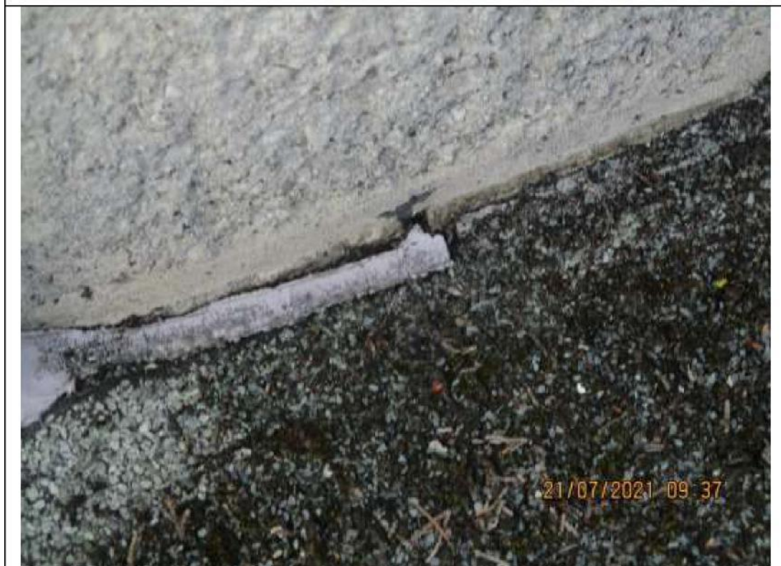
12) Defective mastic to joint of flat roof and window.
