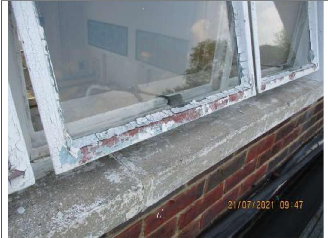
55) Example of flaking paint to original windows.
