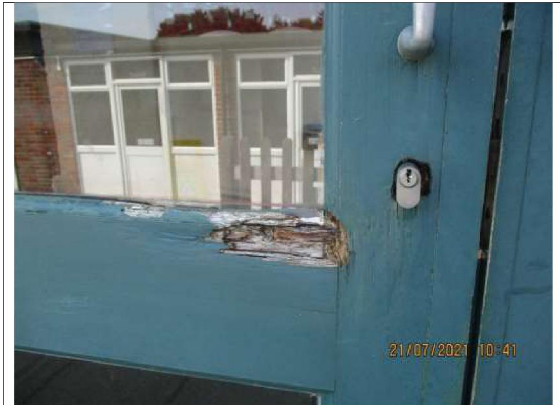
45) Rotten timber door to Year 5/6 block.
