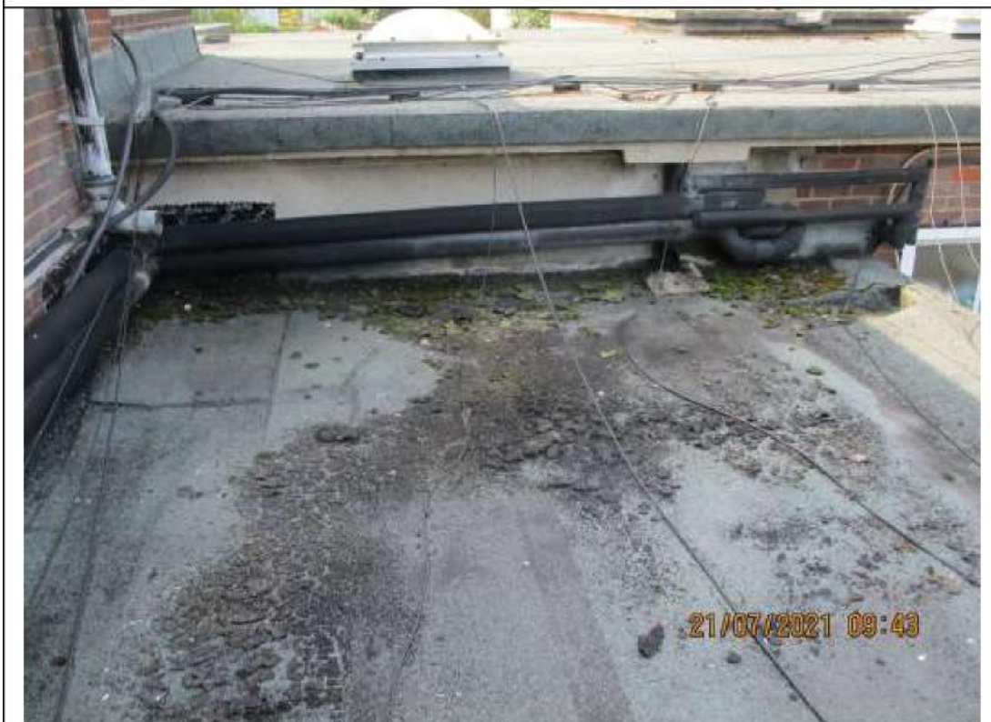
14) Evidence of surface water ponding to flat roof area.
