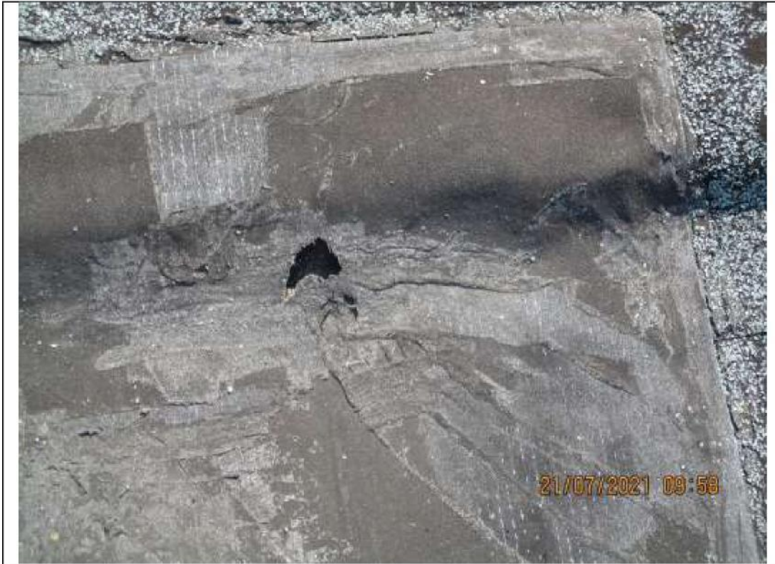
25) Failed patch repairs to link roof to gymnasium.
