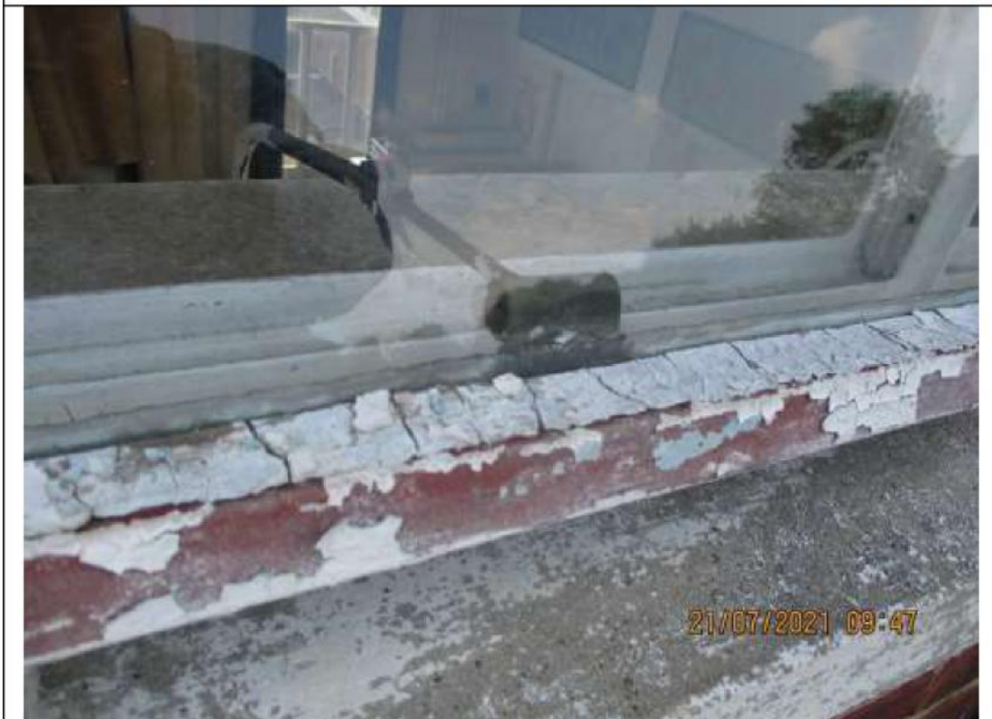
56) Example of flaking paint to original windows.
