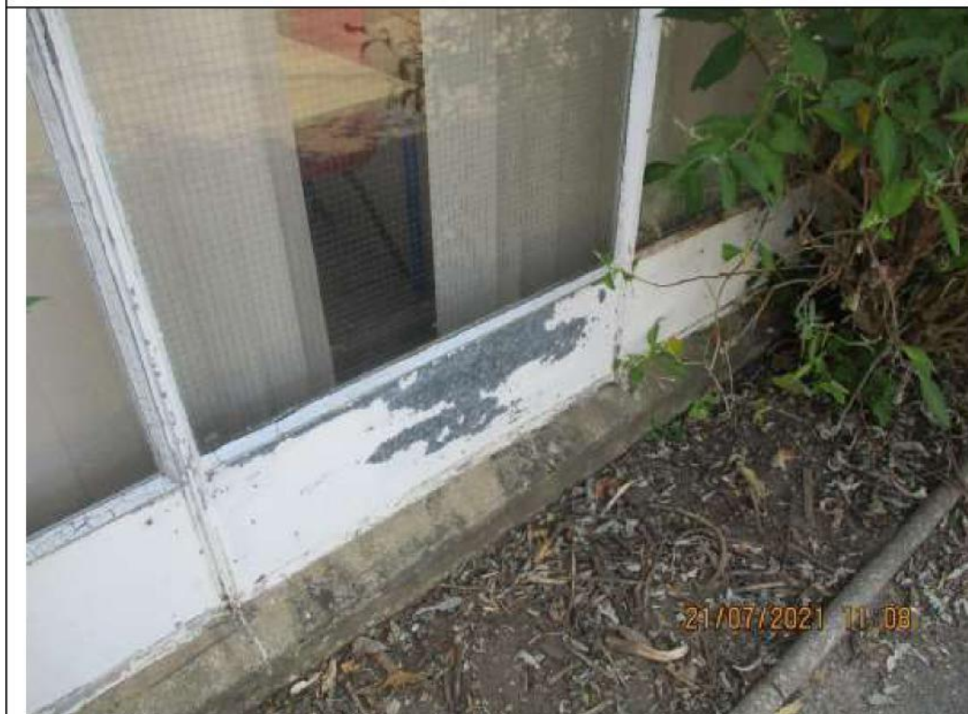
50) Typical flaking and missing paint to original metal door.
