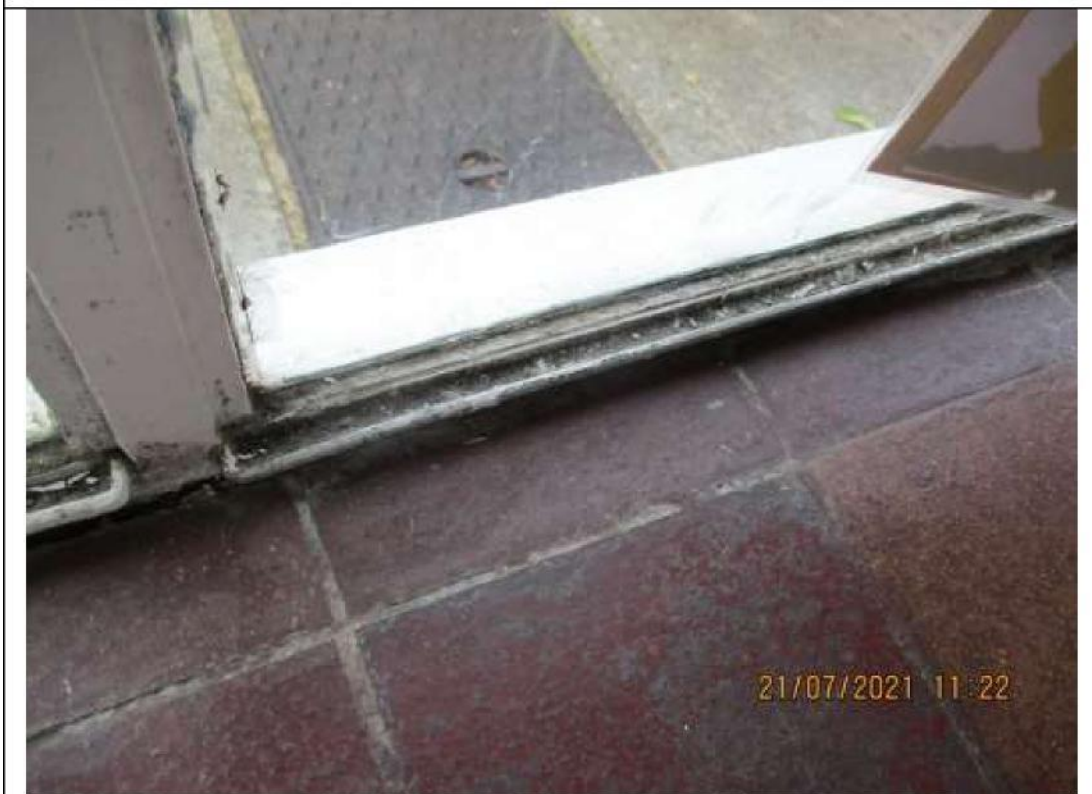
52) Example of internal condensation damp staining.
