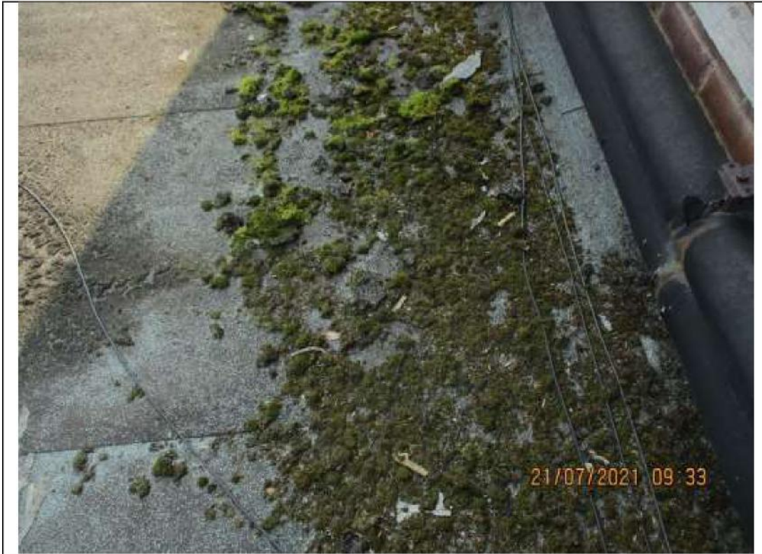
7) Moss build up to roof coverings above KS1 area.
