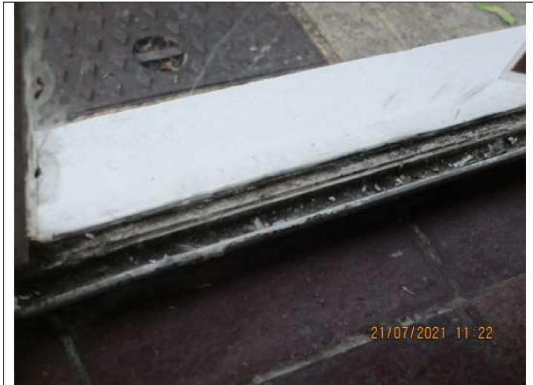
53) Example of internal condensation damp staining to original windows.
