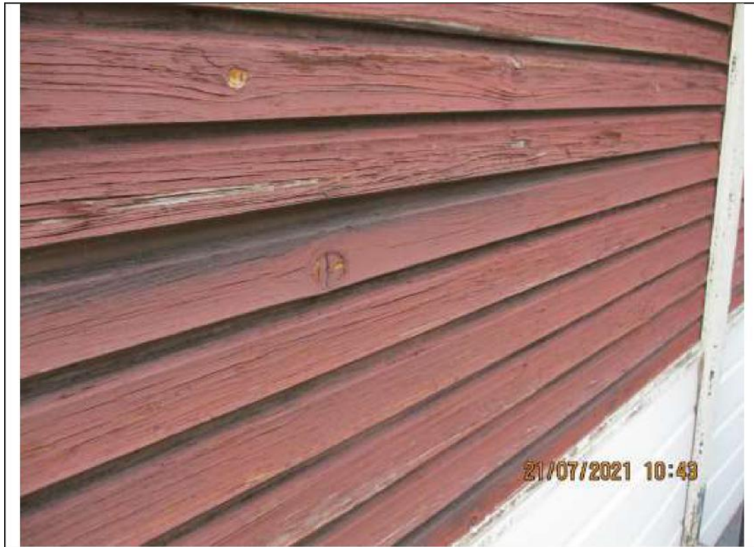
43) Rotten timber cladding to gymnasium building.
