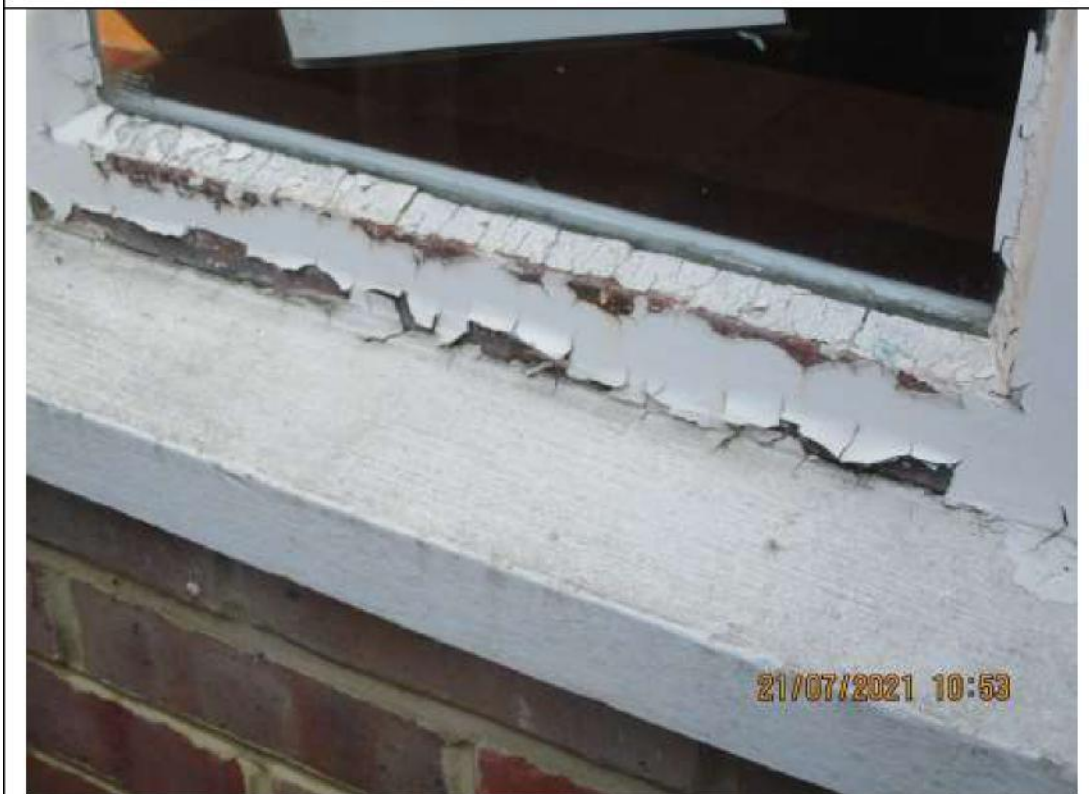
48) Typical flaking and missing paint to original windows.
