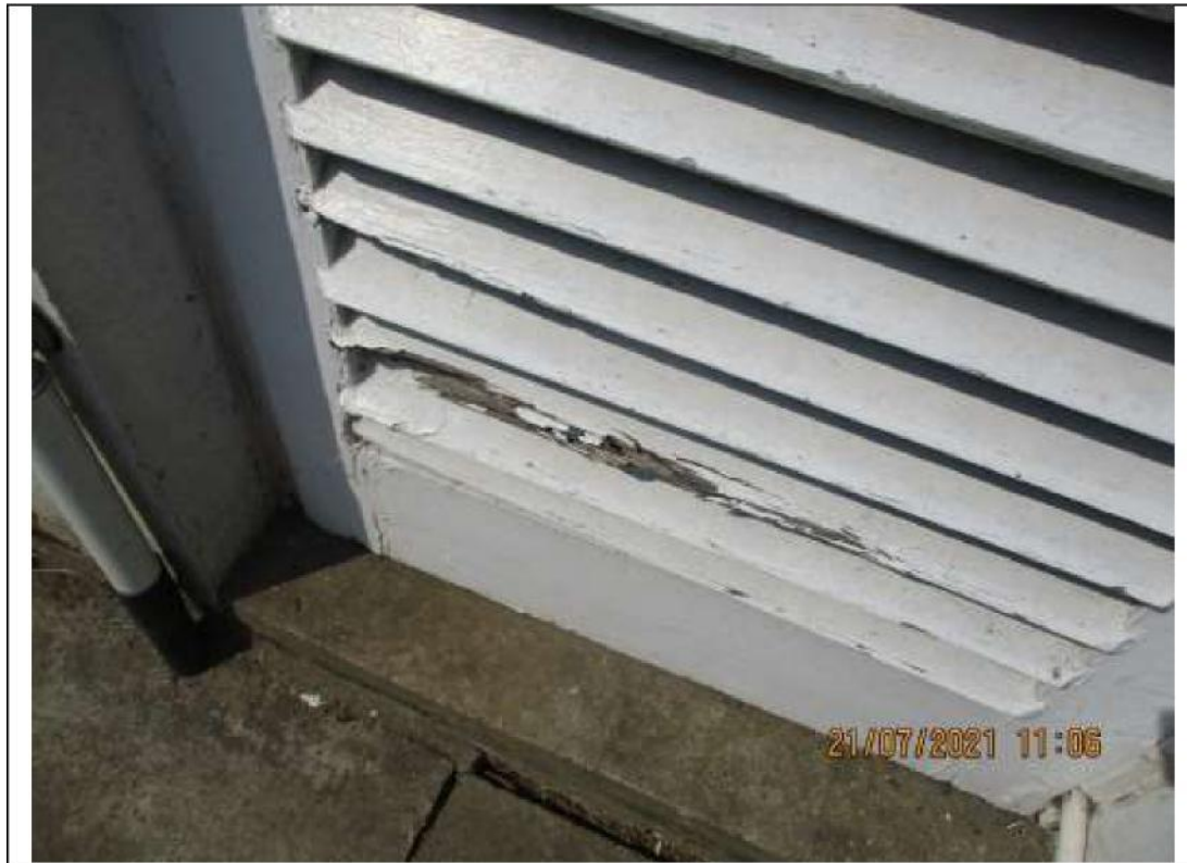
49) Rotten timber louvre door.
