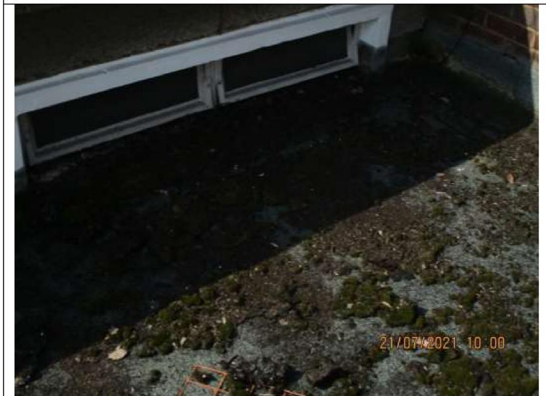
28) Build up of moss to the roof adjacent to the nursery.
