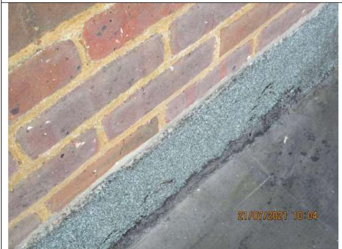
30) Defective upstand detail to link building to gymnasium.
