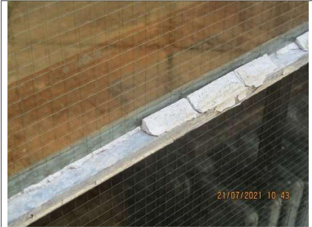
47) Typical cracked and defective window putties to original windows.
