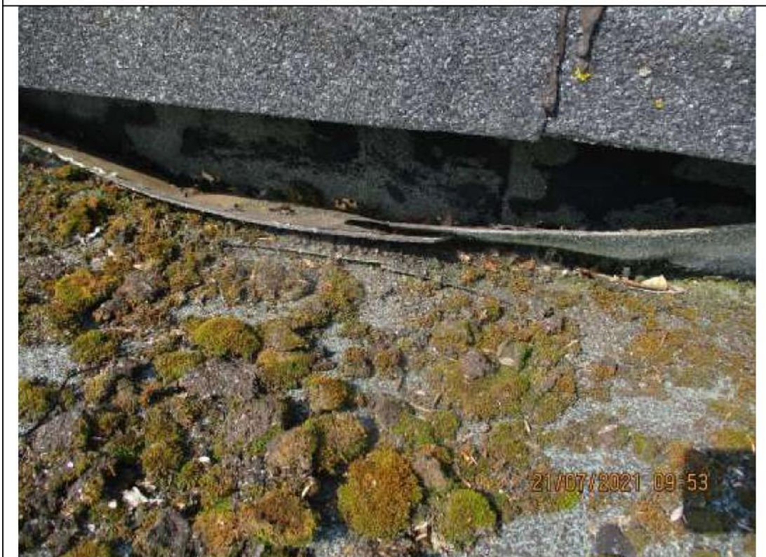
18) Defective felt upstand detail to roof above KS2 area.
