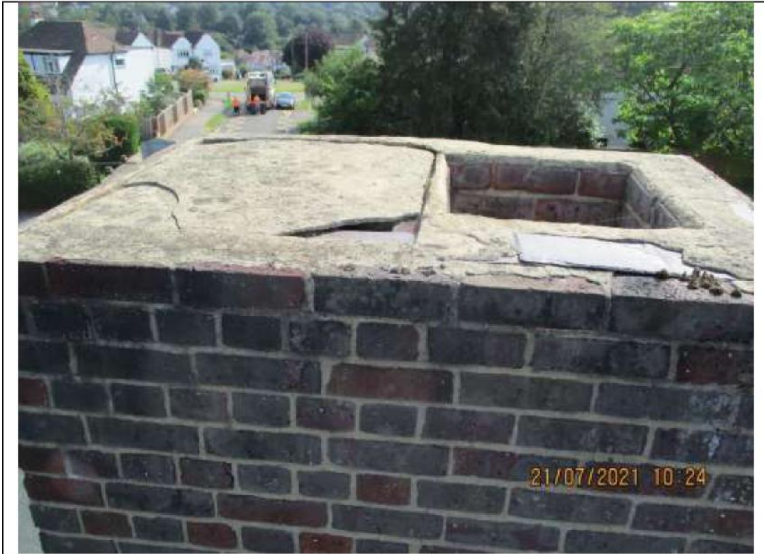
37) Defective stack capping to hall roof.
