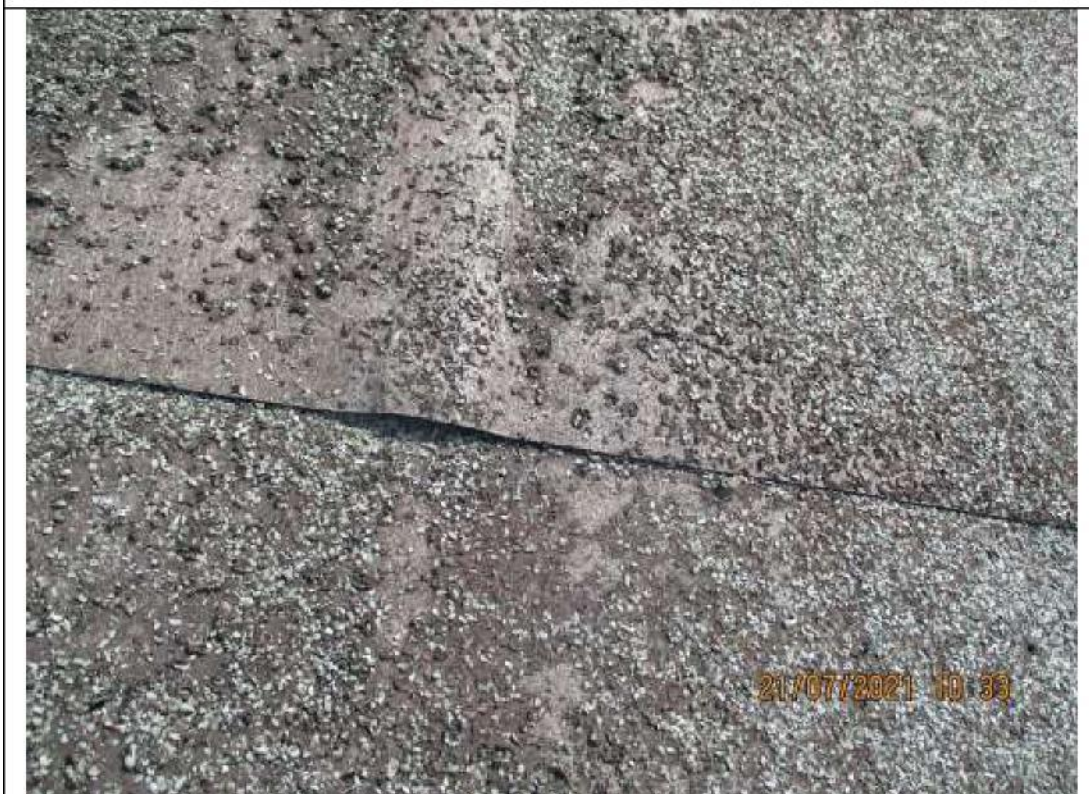
40) Defective/open laps to roof coverings.
