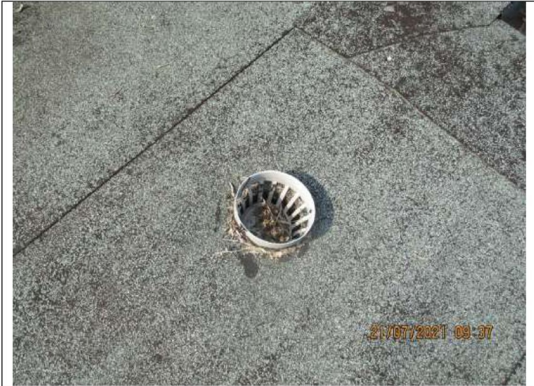
9) Blocked outlet to KS1 area flat roof.
