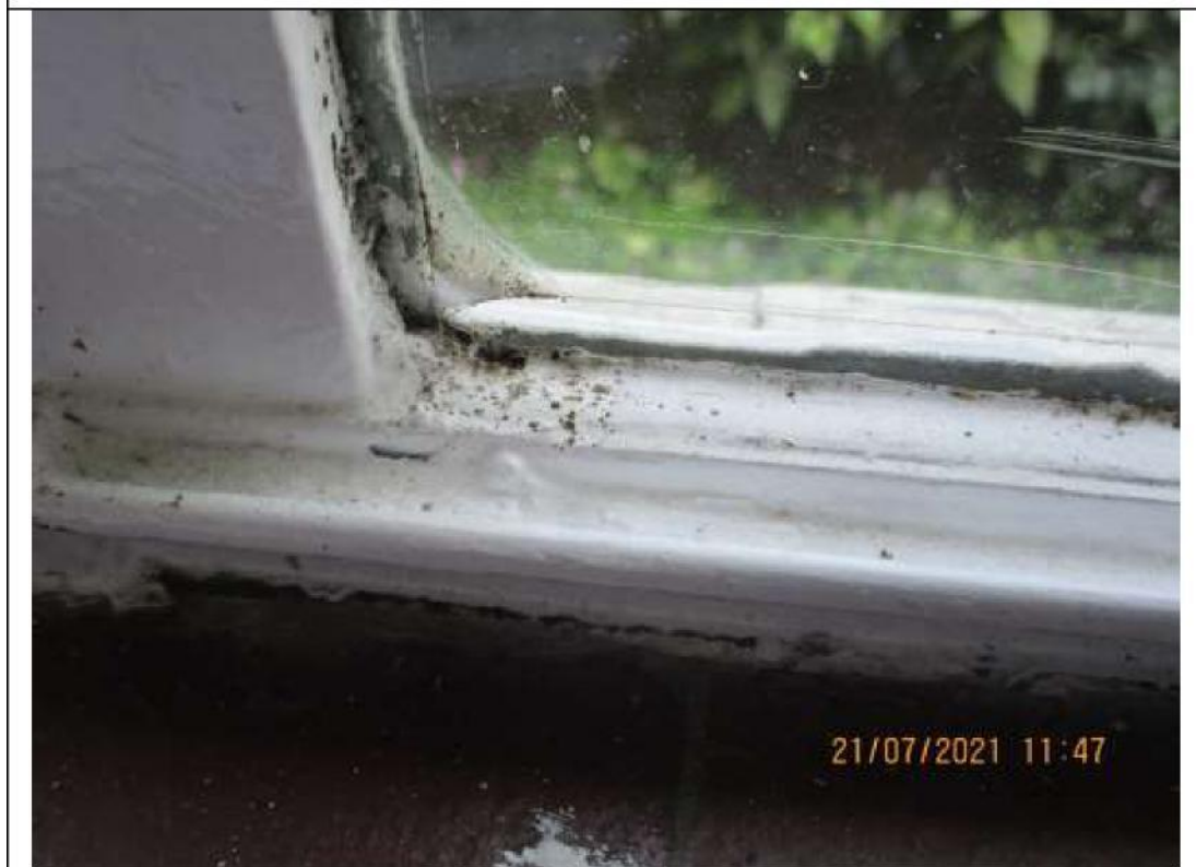
54) Example of mould growth to internal windows.
