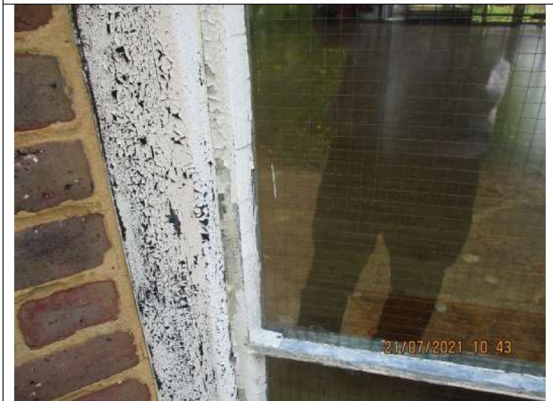
46) Typical defective paint finishes to original windows.
