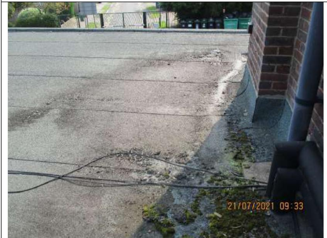
8) Evidence of surface water ponding to lower level roof adjacent to the hall.
