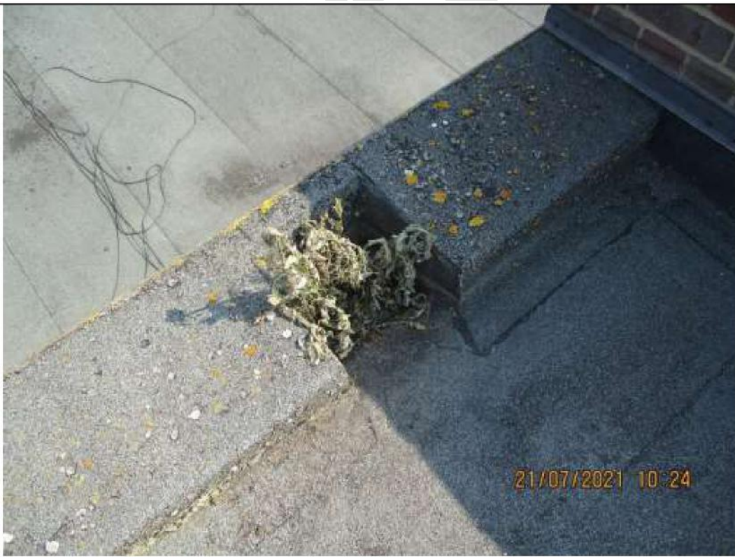
36) Blocked outlet to hall roof.
