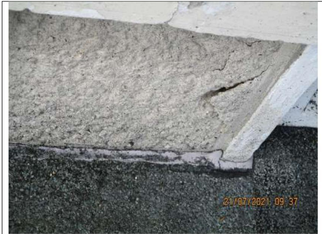
11) Cracked concrete adjacent to windows.
